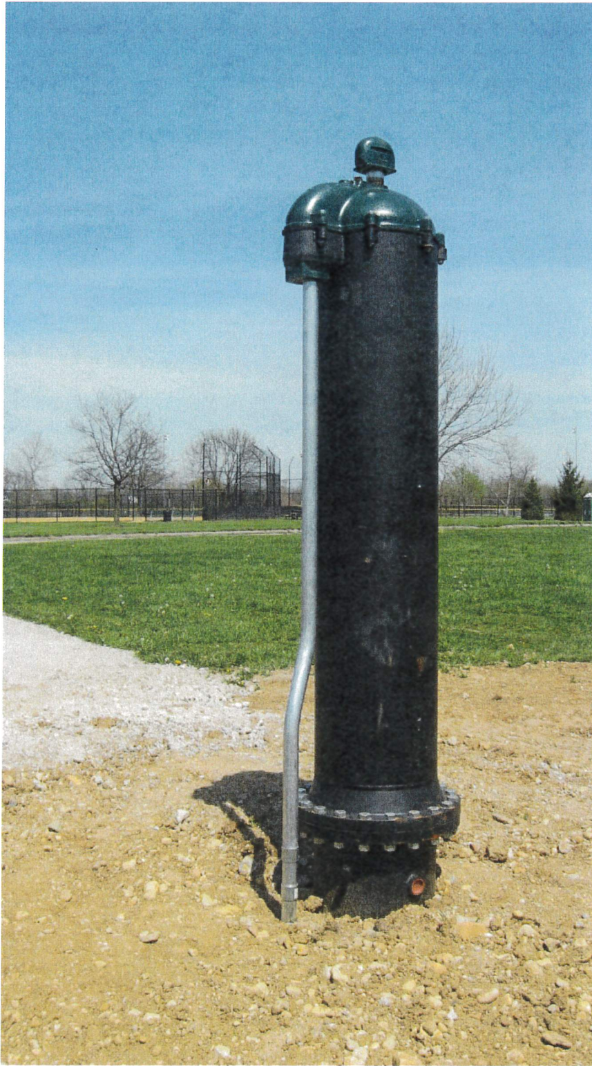
Figure 8. Example Baker Mfg. Pitless Unit as installed on PW-4R.
